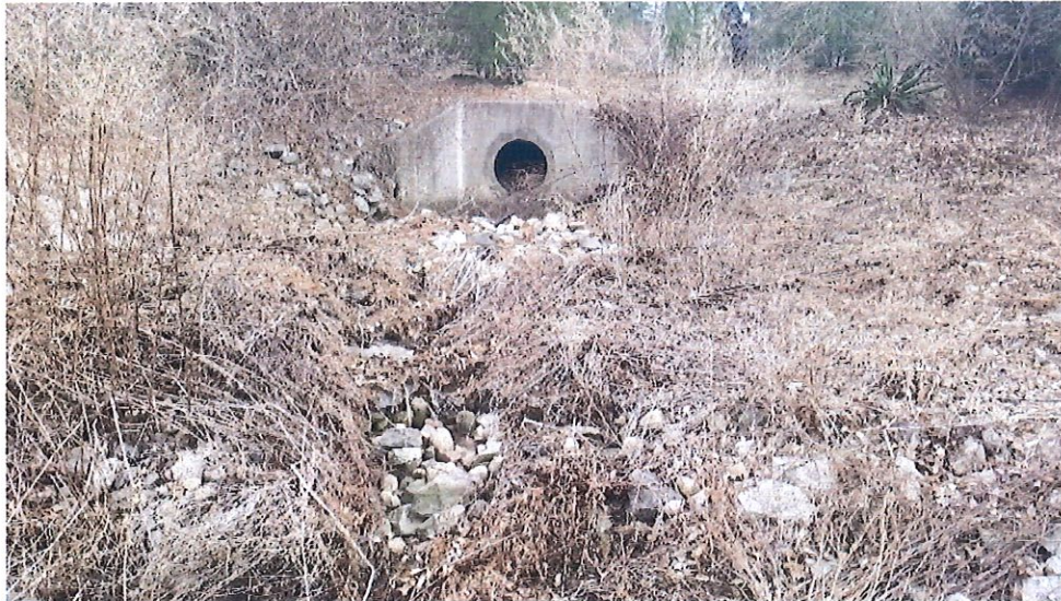
Photo 3: Outfall requiring riprap energy dissipator improvements
