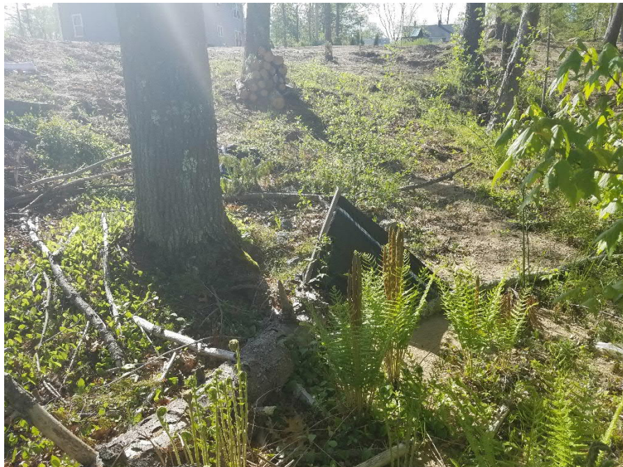
Photo 3: Outfall requiring sediment removal, riprap, and wattles
