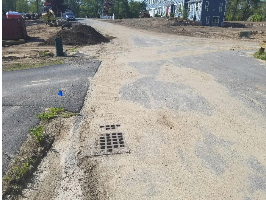
Photo 2: Catch basin requiring sediment removal and inlet protection
