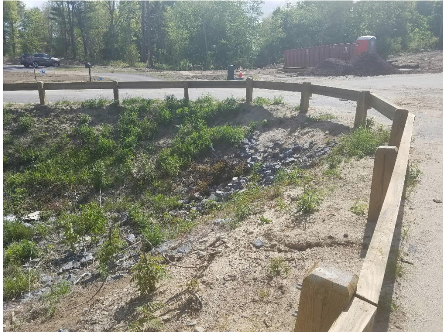
Photo 4: Bioretention basin requiring sediment removal and wattles
